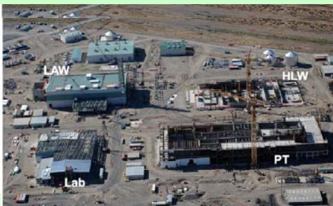
The WTP low-activity waste, high-level waste, pretreatment, and analytical laboratory facilities under construction
